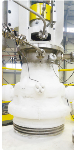
Cryogenic Pump (VS6)
